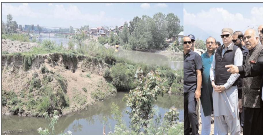
the breach site.
